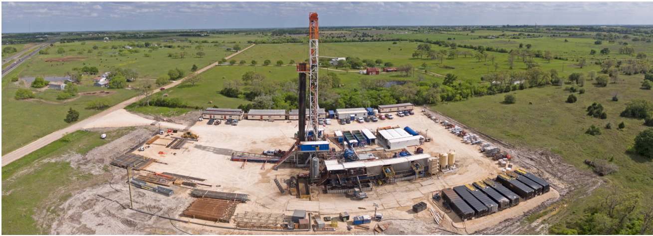
Figure 2. A drilling rig operation for a shale formation in Texas shows the extent and scale of some of the infrastructure. CREDIT: Shutterstock via Photographer: Jeffrey M. Phillips.
