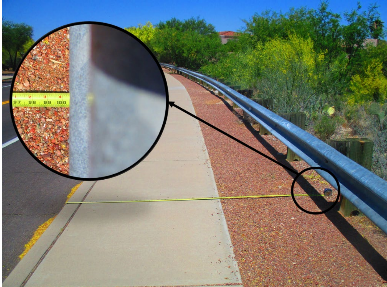
Figure 9. Measuring CDIST, this longitudinal barrier has a curb offset of 8.4 feet (101 inches).
